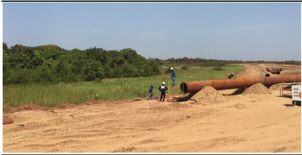
Figure 3.77 Installation works in progress in the central section of the GAC platform
