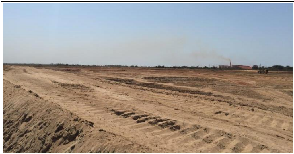
Figure 3.76 General view of the cleared area in the inland section of the GAC platform
