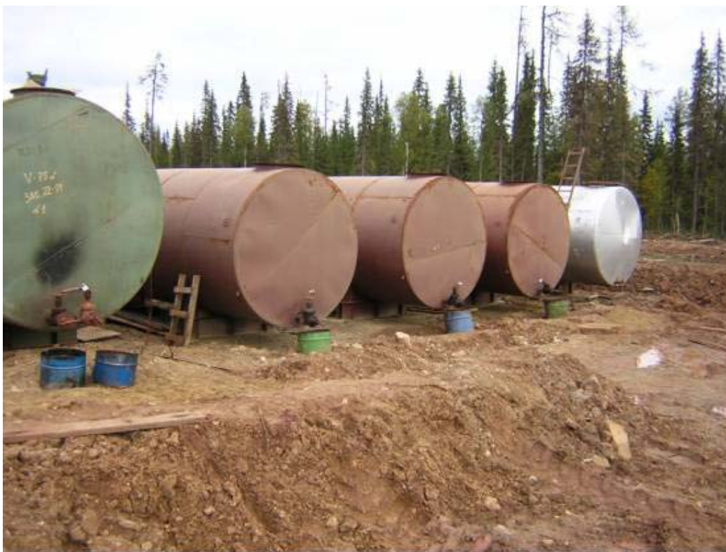
Plate 20: Fuel storage tanks at the mine indicating the lack of spill protection infrastructure
