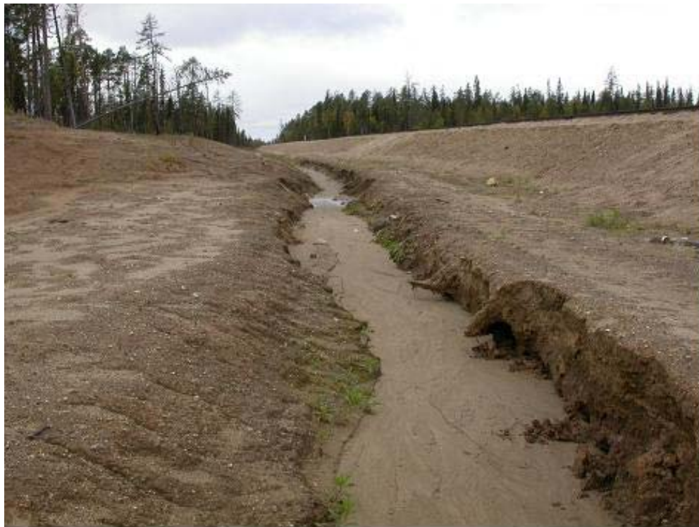
Plate 7: Erosion of unvegetated road embankment
