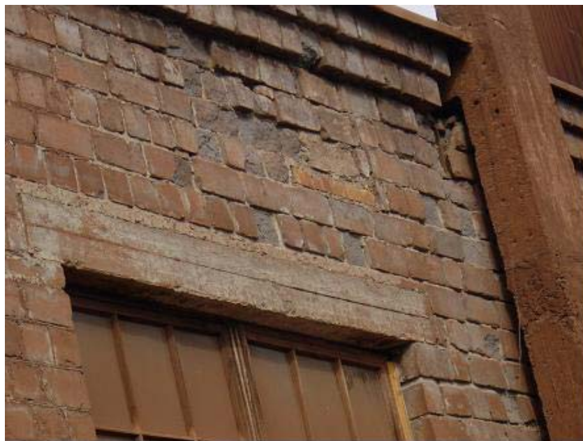
Plate 25: Evidence of brick corrosion on buildings at UAZ
