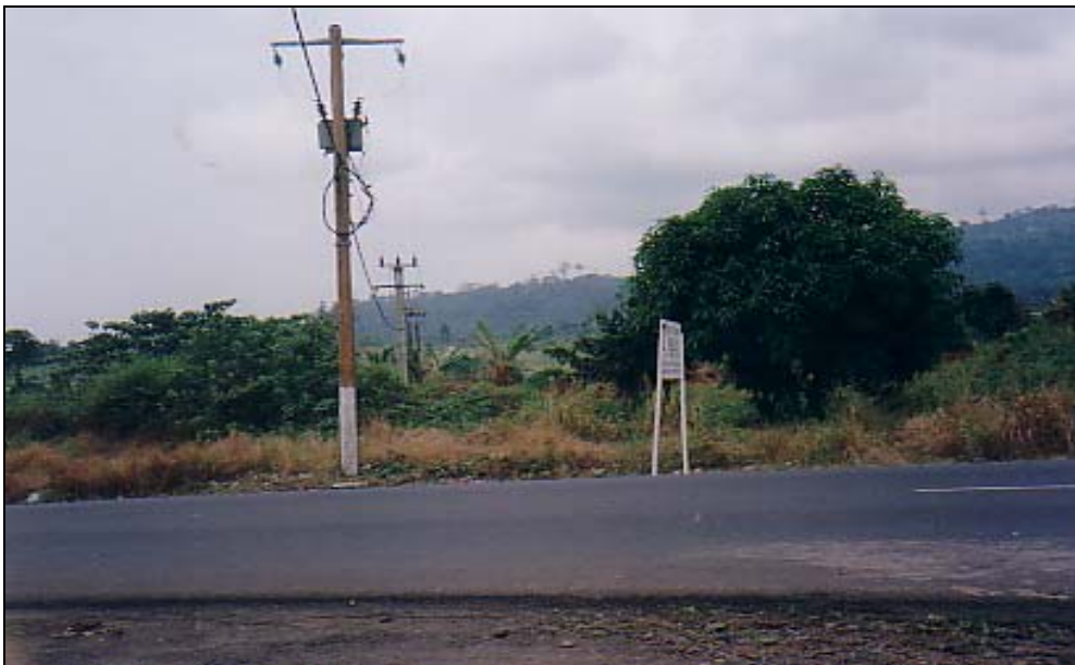
Figure 3 – View of the Proposed Line Route from the AES-SONEL Substation in Limbe
