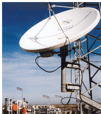
Satellite communication system
