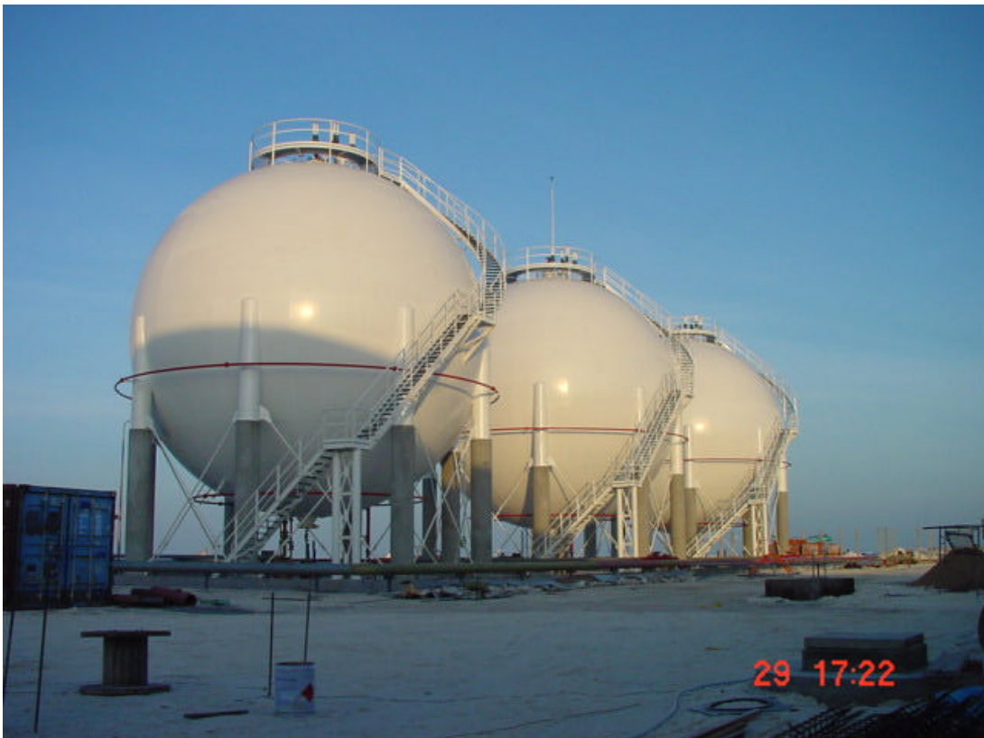
Photo 4 North – LPG storage spheres at Villa Hakatha
