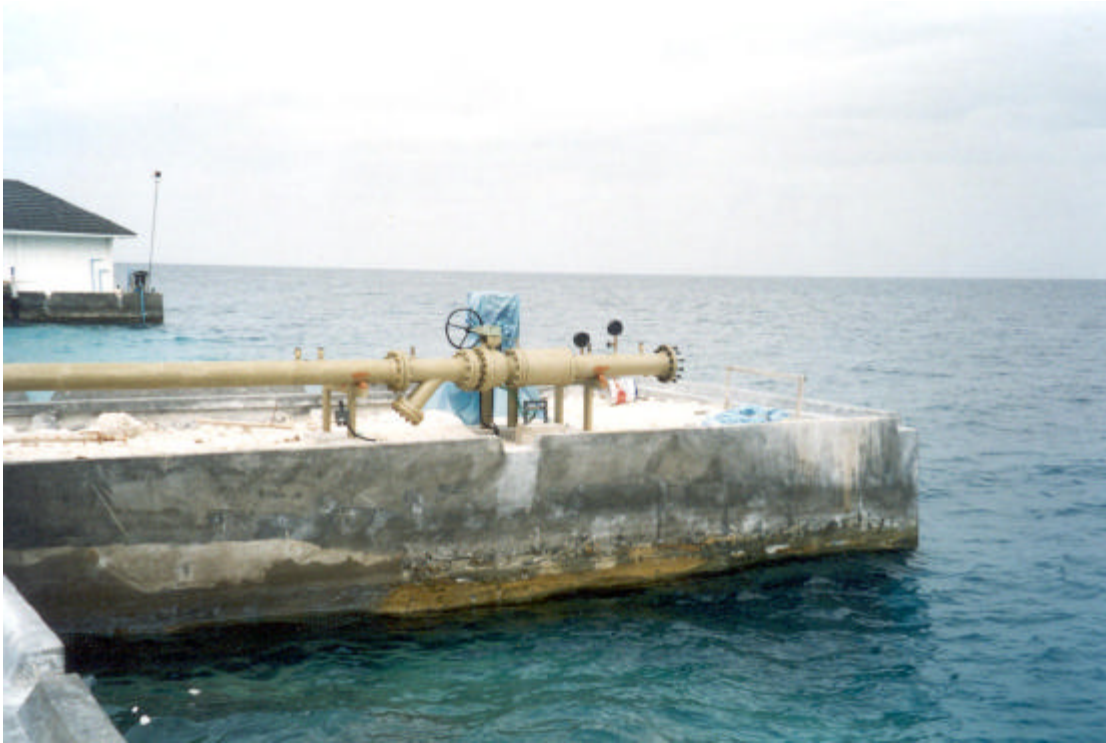
Photo 3 North - Open Sea showing the LPG pipeline on jetty
