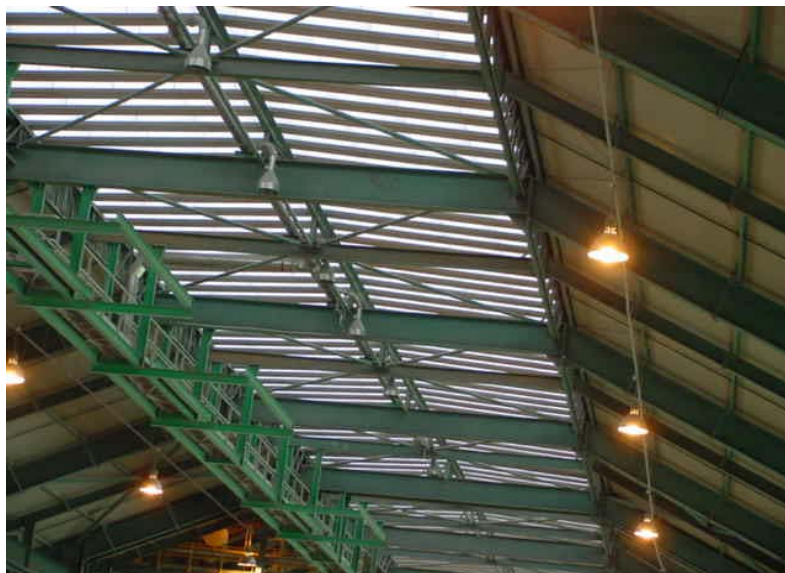
Figure 4: Photograph showing potroom roof vent monitoring system.
