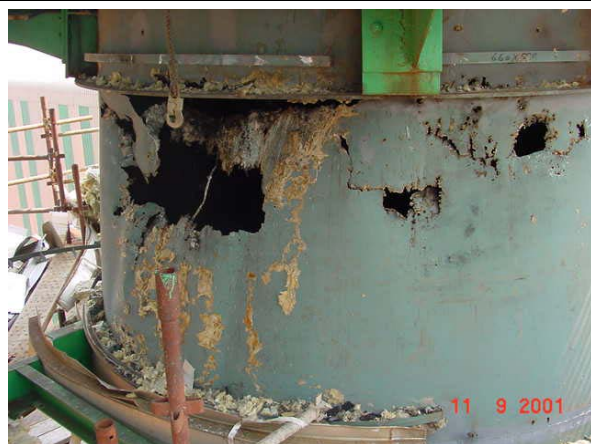
Figure 1: Corrosion on the damaged section affected the walkway structure as well as the shell.
