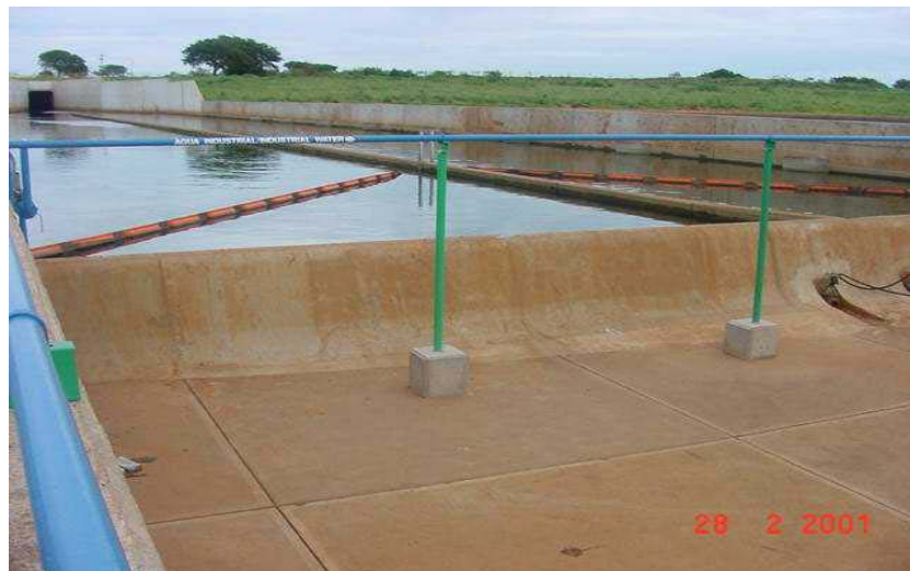
Figure 5: View of the impoundment dam inlet structure (stormwater enters the inlet from the far side). The inlet provides for sediment trapping and oil skimming. The complete impoundment dam can be seen in the cover photo of the entire smelter site.
