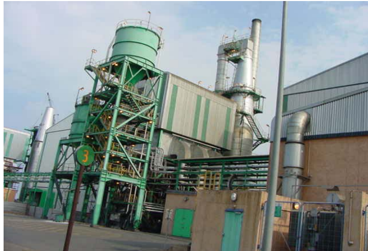
Figure 3: Photograph showing fume treatment centre at carbon plant with second unit under construction in background
